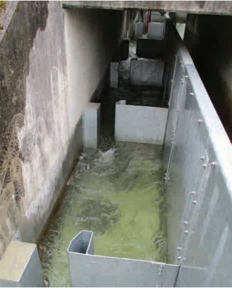
The new fish ladder
