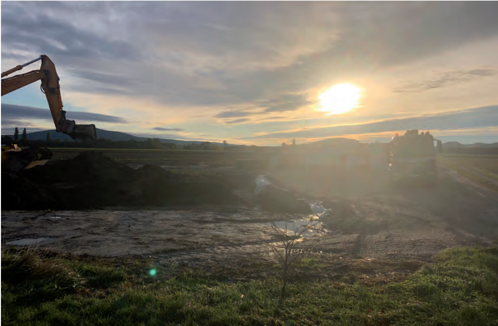
Deep well tank Engelhartstetten: Morning ambience at the beginning of the cutting of the pit for the deep tank.
