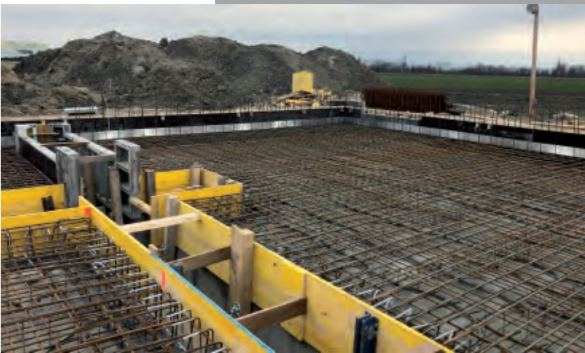
Deep well tank Engelhartstetten: currently under construction. Reinforcement and concrete works on the base plate.
