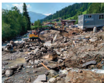
Disastrous damages of the infrastructure at Kelchsauer Ache river, Tyrol
