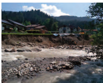
Massive bank crack of several meters in height with a temporary protection of the energy supply at Kelchsauer Ache river
